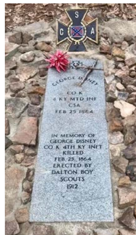
Left to right: Spreading concrete mix; placing new headstone; and the newly refurbished grave.
