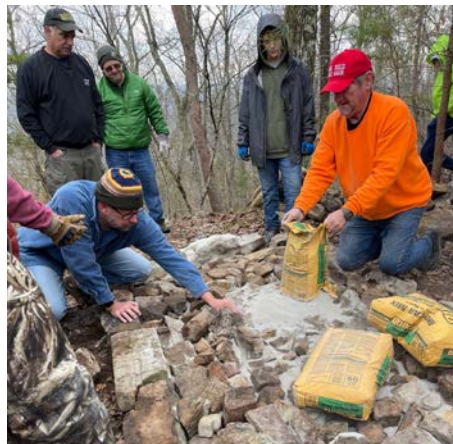
Left to right: Replacing and rearranging rocks for a more level surface; preparing concrete mix on rearranged rocks. In the photo at right, Bob Jenkins, who provided the recent photos, is in blue on left, placing a rock.
