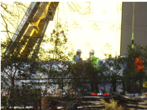
AHC's Gordon Jones (left) and Jackson McQuigg inspect scroll 2 before placement in new building.
