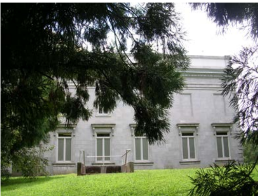
North face of current building. Ground will be excavated and wall will be removed to right of stairwell. Texas and tender will be rolled out on temporary rails and loaded onto trucks.
