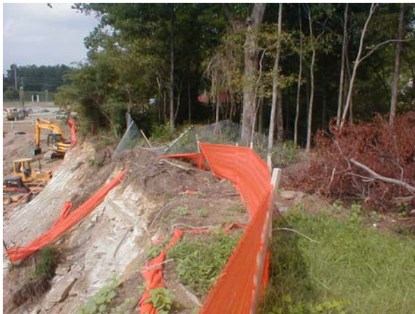
The damage discovered on 26 August.
