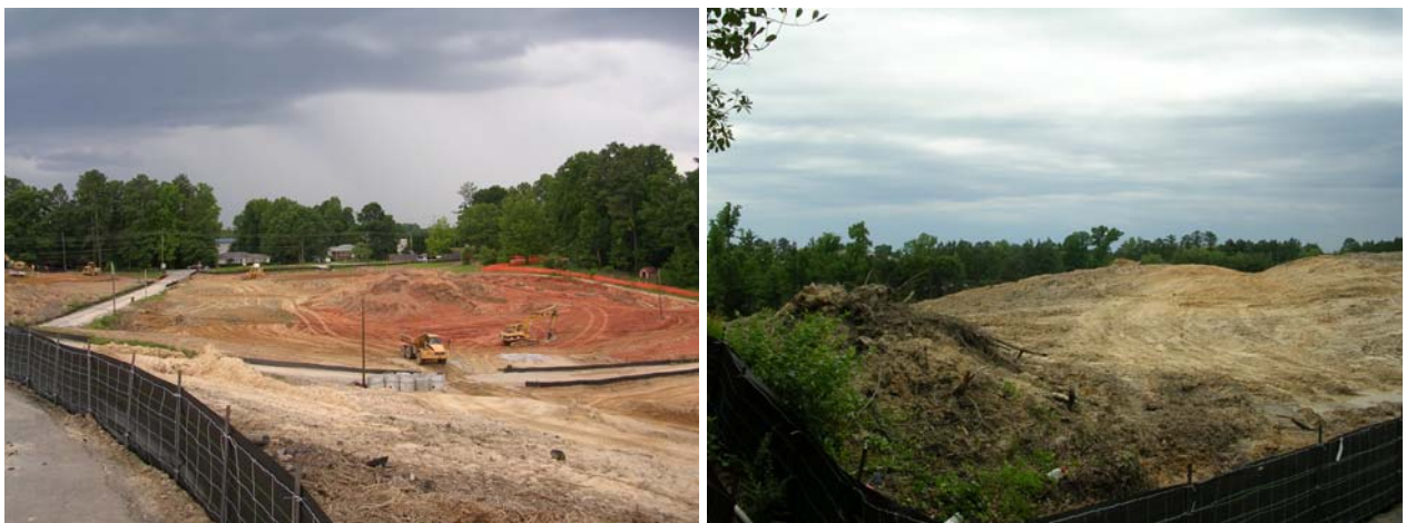
Looking west from current curve in Fort Drive. Looking south at former site of redan (item 6). Beech Street runs south to north across photo.
